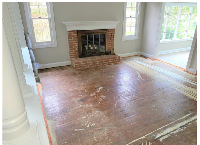
1st Floor Family Room after carpet & padding removal and surface HEPA Cleaning and Disinfection
